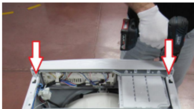
3.10. Tighten two screws fixing control panel.
