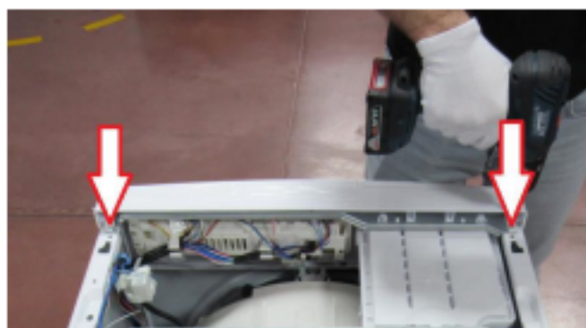
3.10. Tighten two screws fixing control panel.
